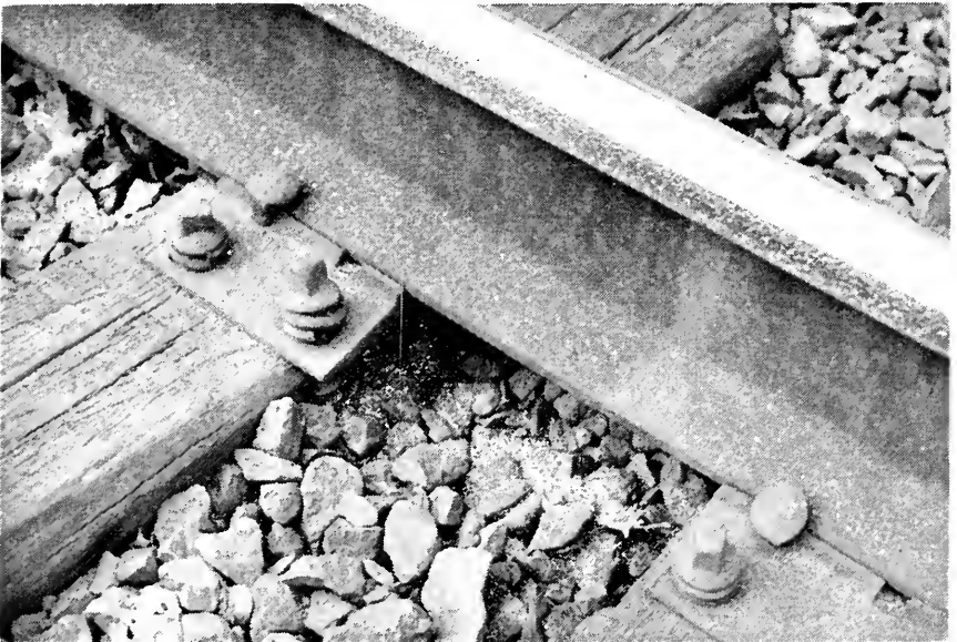
Fig. 2—High rail on 7-deg 30-min curve. Note metal flakes on rail base, tie plates and ballast.
